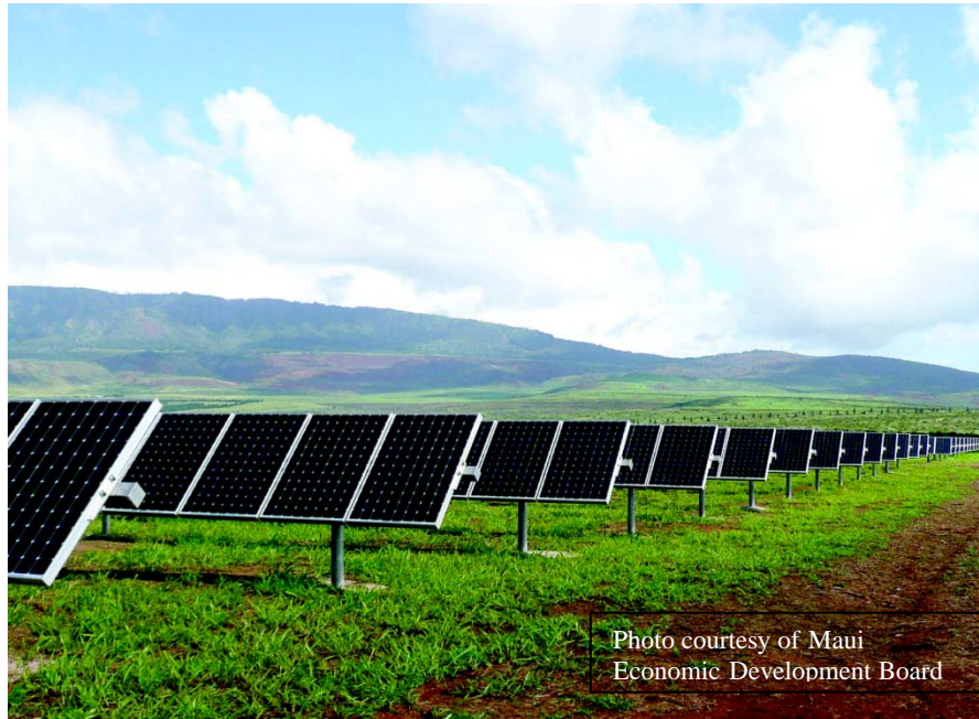
Figure 3. La Ola Solar Farm, Lanai features 7,400 photovoltaic panels that tilt to efficiently track the path of the sun and is remotely controlled by Maui Electric Co.
