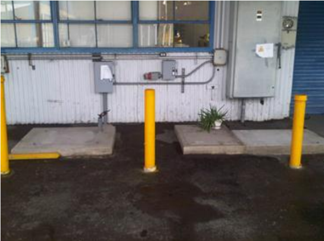
Figure 5: HCATT Charge Spot site (Before)
